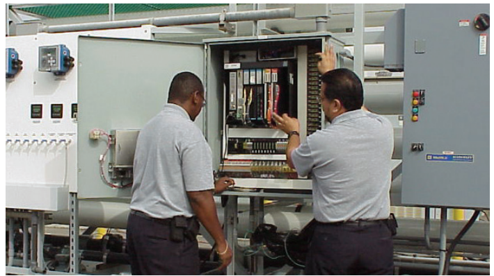
Photographs courtesy of Long Beach Water Department.
